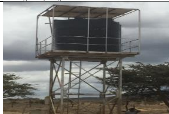
Ilkioriti community = borehole fitted with solar pump
